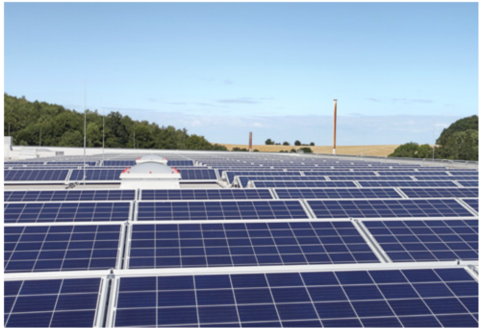
Photovoltaic system on the roof of our headquarters in Mühlthal.
